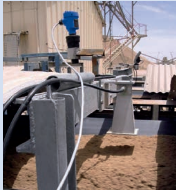
Moisture measurement of phosphate - LB 567 with horn antennas in combination with an ultrasonic height sensor in order to compensate for the varying bulk material heights.
