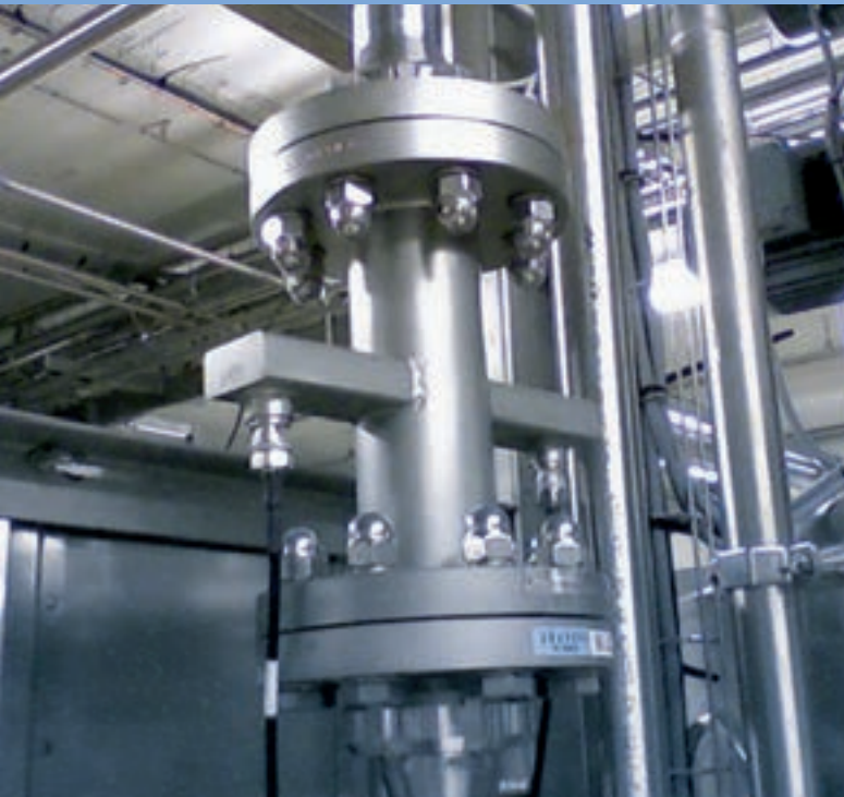
Determining the dry substance in a wastewater pipe – LB 566 with flow cell.
