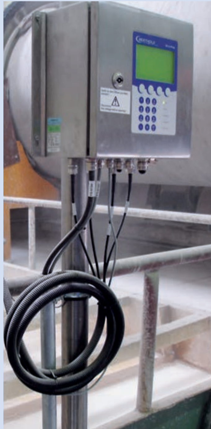
MicroPolar installation in a power station for measuring the concentration of a limestone suspension
